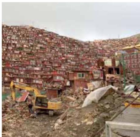
Demolition at the important religious institute of Larung Gar in Serthar, Sichuan (Kham, eastern Tibet) began last week with images appearing on social media in China, and netizens expressing concern and distress.
